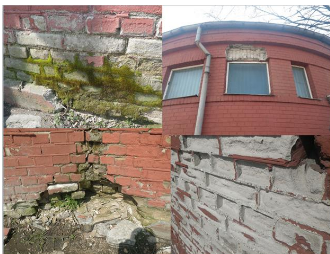
Fig.2. Damaged building envelope elements
